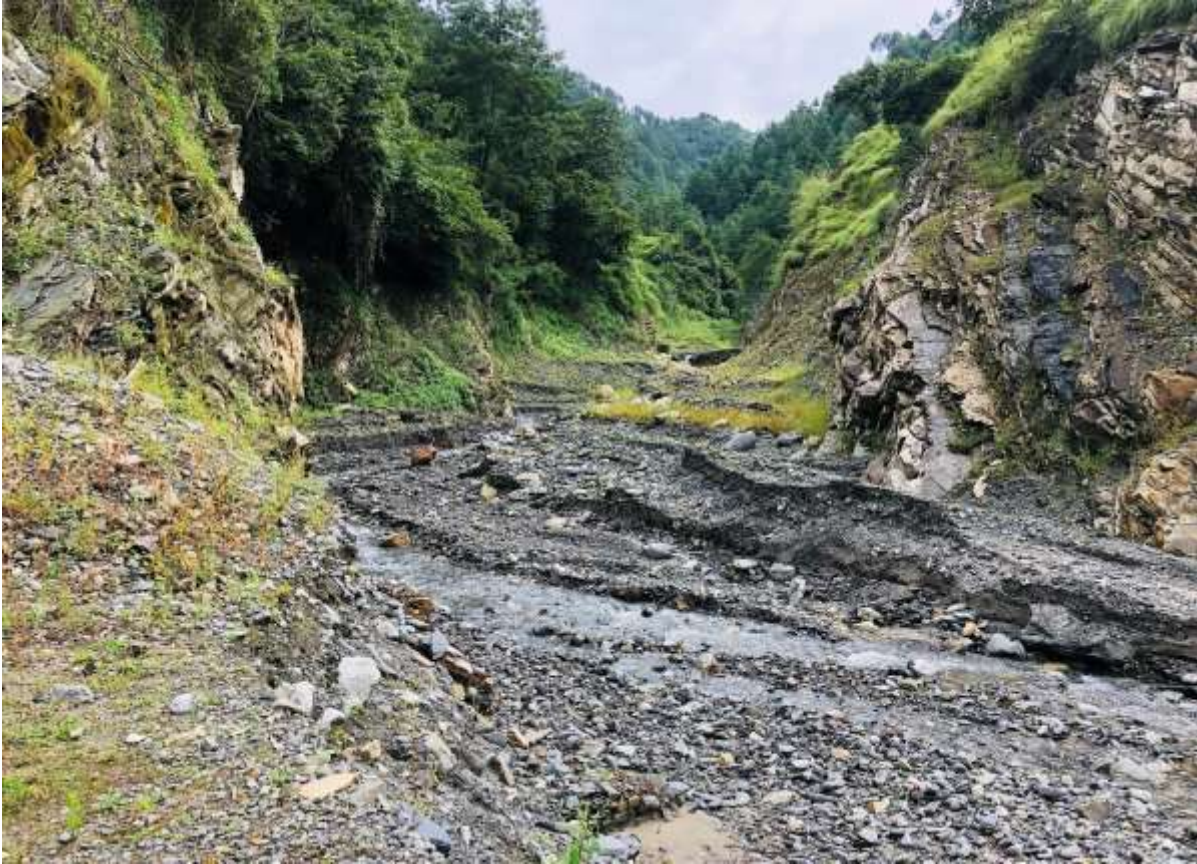
Figure 11: A debris flow occurred due to unmanaged slope after excavation and lack of control measures prior to the failure
