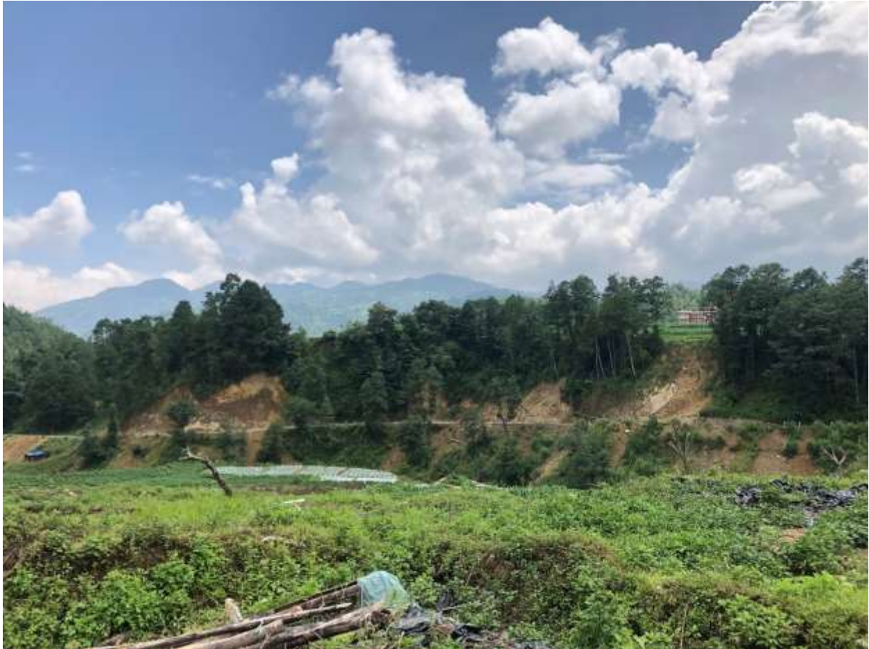
Figure 15: Road-cut failure observed at Sarbang area
