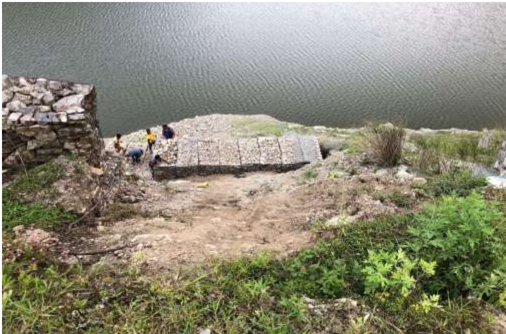
Figure 17: Gabion works undergoing in an active erosional failure on loose sediment slope
