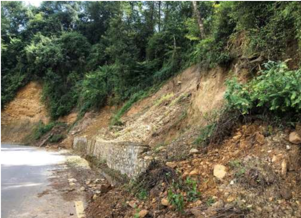
Figure 13: Landslides along the road
