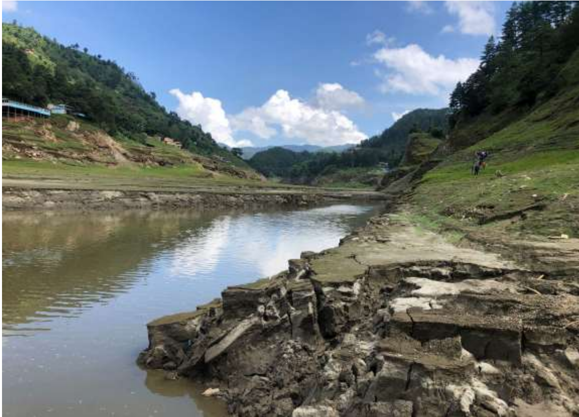
Figure 6: Recent undercutting by the flowing water courses
