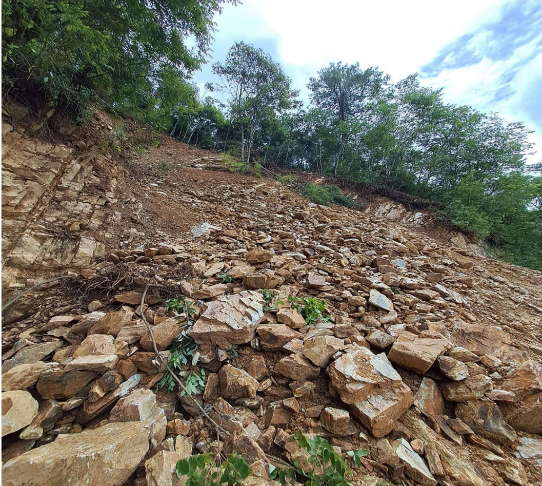
Figure 12 Chitlang Kharga Landslide
